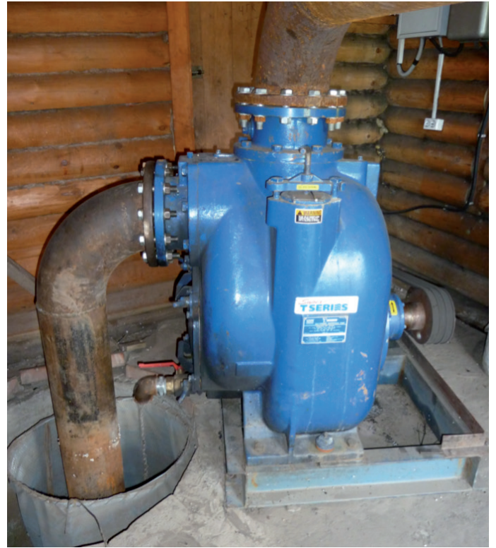
Gorman-Rupp super T8 pump for priming the water from the lake
