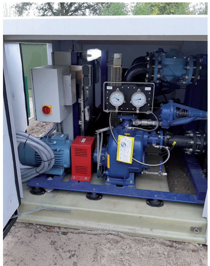
Interior sewage booster pumping station.
